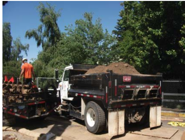
All materials excavated for the bore pit and outfall were temporarily stored and then reused in the project.
