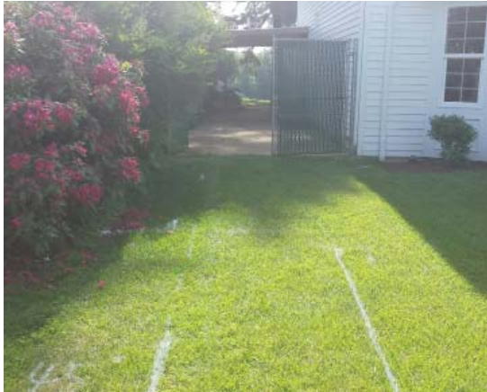
The new storm drain needed to be placed directly under existing carports and mature landscaping.
