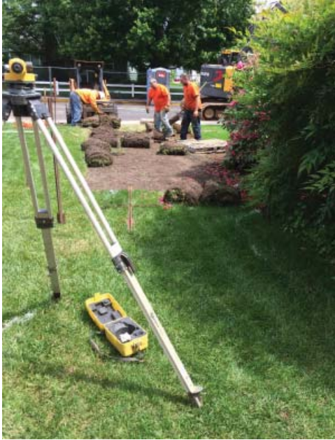
The City made good on their promise to replace turf that was disturbed during construction.
