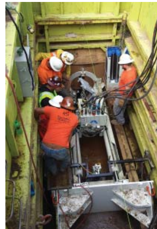
The boring equipment fit snugly in the bore pit. The team successfully bored the smaller pilot bore and then placed the larger 20-inch steel casing - all within one weeks time.
