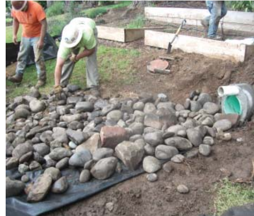
The existing and new outfall locations were located in the floodplain. Special measures were taken to control potential erosion and confine the work area.
