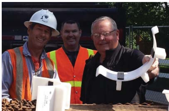
Plastic spacers were used inside the casing to precisely position the storm drain line.
